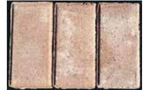
Pavers with efflorescence
